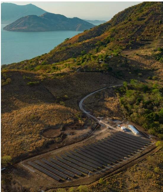
Figure 11: A solar-plus-storage plant serving the Meanguera del Golfo region
